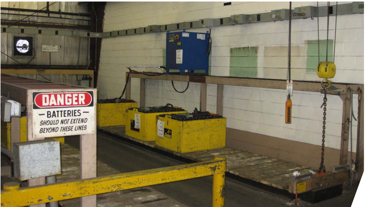
Battery charging area
